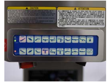
Back lit back-up controls for emergency situations
